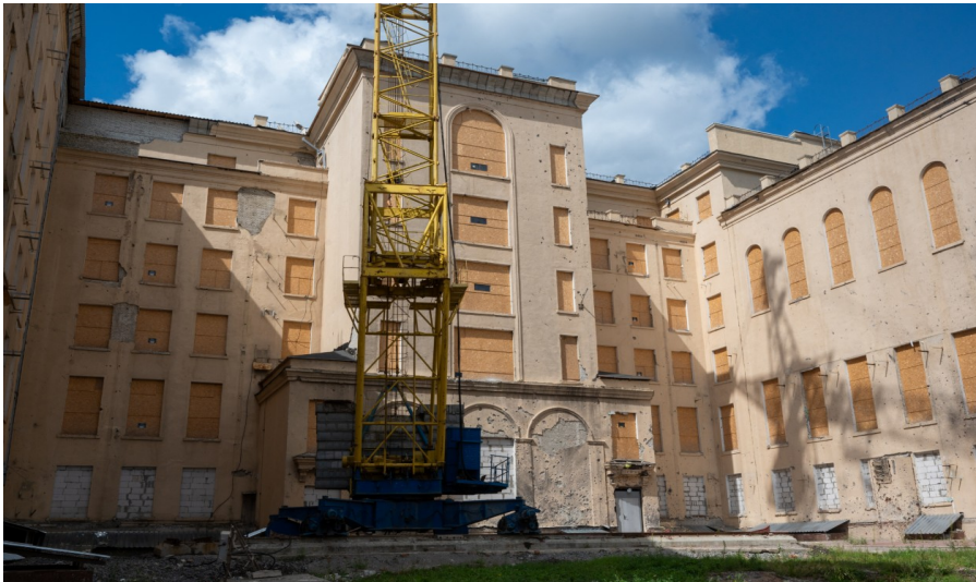
Fig. 4: Preservation of the Kharkiv Regional State Administration Building after the Russian missile strike (Sergiy Bobok, August 23, 2023). Photo via Wikimedia Commons.
